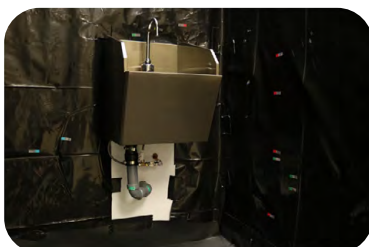
Trough sink and short automatic sensor faucet
