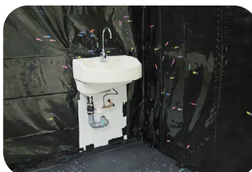
Barrier-free sink and short automatic sensor faucet
