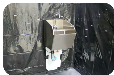
Trough sink and tall automatic sensor faucet
