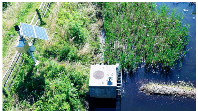
Figure 4: SmartSWM as Applied at Century Engineering Headquarters. Reproduced with permission from Century Engineering.
