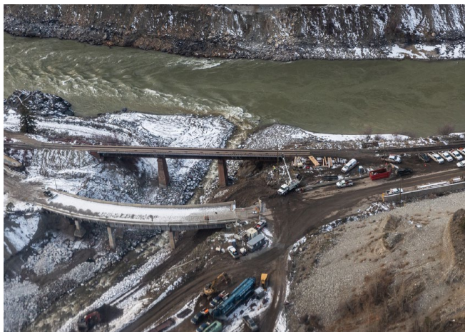
Figure 8: Bridge washed out from atmospheric river in Merritt, BC, 2021. Source: Province of British Columbia.
