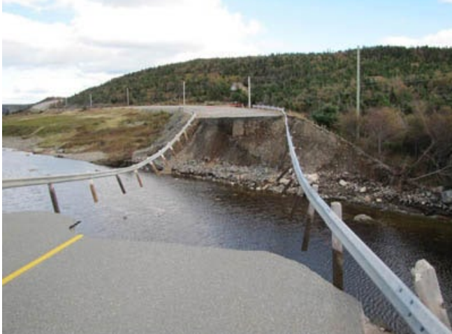
Figure 6: Highway damage resulting from Hurricane Igor, 2010. Source: Environment Canada.
