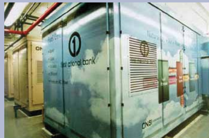
Four UTC Fuel Cells 200kW power plants now provide the primary power source for the First National Bank of Omaha.
